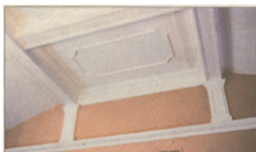
A coffered ceiling covers beams that needed recurring repairs in this Annadale home, where pilasters built on the walls support the new work. Crown molding was added to complete the renovation by Home-works Contracting of Richmond. PHOTO COURTESY OF JACOBSON CONTRACTING INC.
